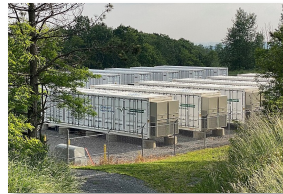
Battery farms 1,2 GWh ↑
