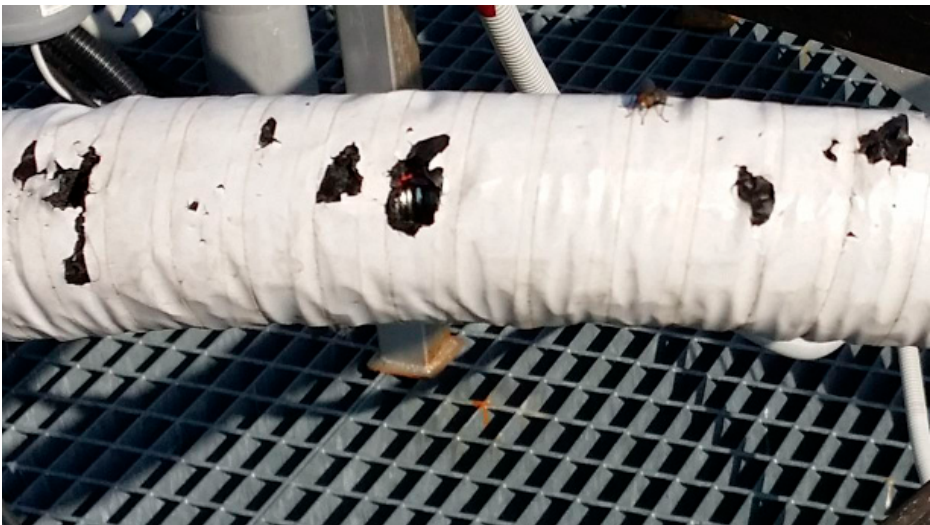
Joonis 5. Linnude poolt kahjustatud juba eelnevalt parandatud soojuskandja toru isolatsioon Figure 5. The insulation of the heat carrier pipe which was previously repaired has been damaged by birds
